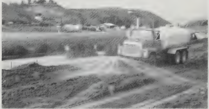
Figure 6.18 A water truck spraying a new lift of soil for a fill and preparing it to be compacted.
