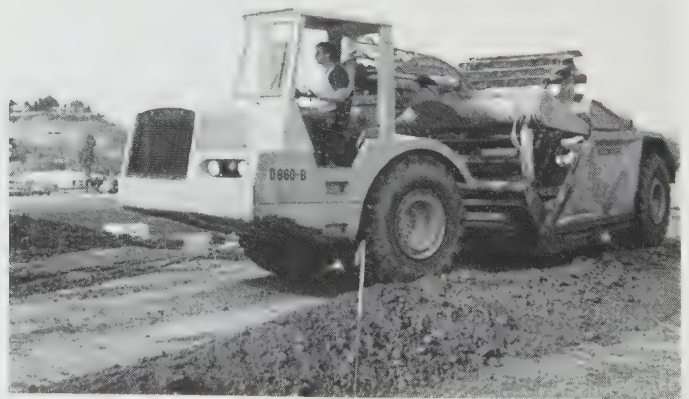
Figure 6.11 A scraper transporting a load of soil across a construction site. This scraper is equipped with an elevating mechanism at the front of the bowl to assist in loading soil.
