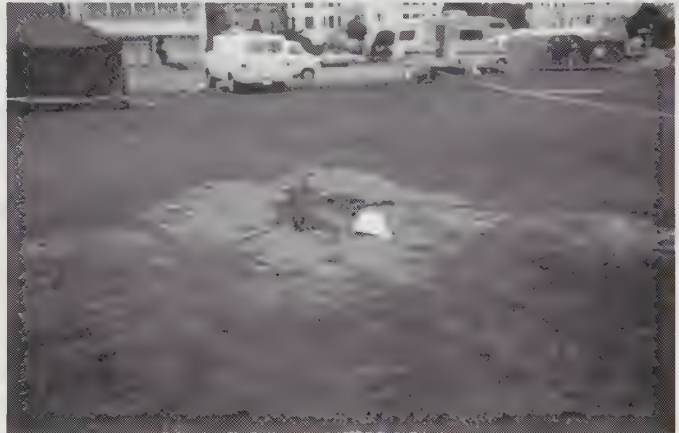
Figure 20.7 Sand boil in Marina Green, San Francisco, California, as a result of the 1989 Loma Prieta Earthquake. The green is underlain by a sandy hydraulic fill (Earthquake Engineering Research Center Library, University of California, Berkeley, Steinbrugge Collection)
