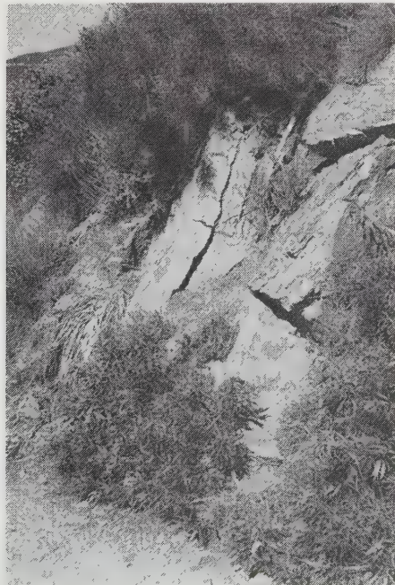
Figure 2.5 Steeply inclined bedding planes in a sedimentary rock. Shear failures can easily occur along such steep planes, especially when excavations destabilize the adjacent ground. For example, the rock in the foreground has already moved along one of the bedding planes, and has become twisted out of alignment.
