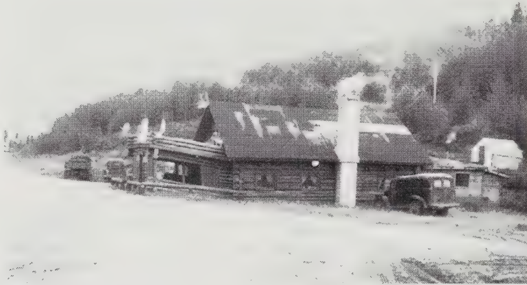
Figure 18.6 Heat from this lodge in Alaska thawed the permafrost below, causing it to settle. However, the permafrost did not thaw beneath the unheated porch (Photo courtesy of Professor Richard L. Handy).
