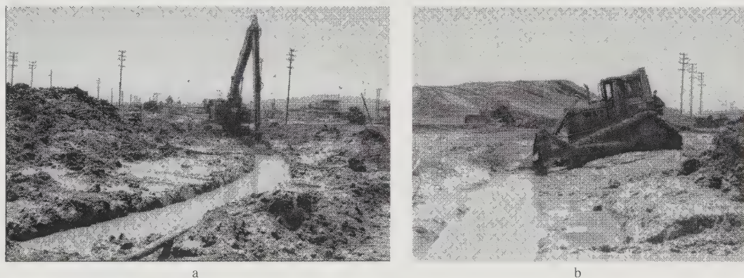
Figure 8.32 A slurry trench barrier under construction: a) An excavator is digging the 20 m (65 ft) deep trench through a slurry, b) then a bulldozer pushes in a clayey backfill.
