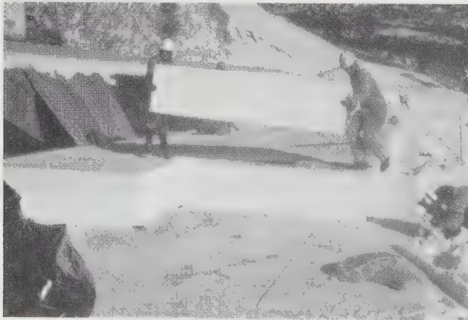
Figure 6.39 Geofoam blocks being placed to produce a lightweight fill for a highway in Colorado. (BASF Corporation)
