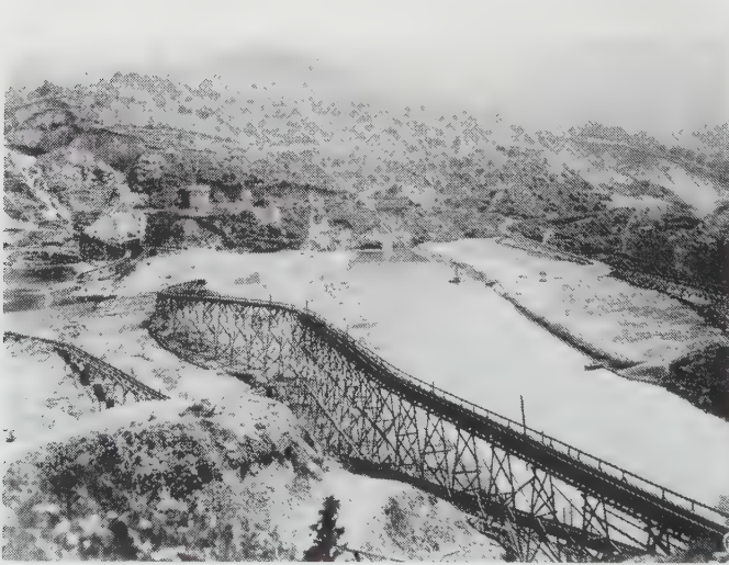
Figure 6.5 Construction of San Pablo Dam in California using hydraulic fill techniques, circa 1918. Two fills are being placed simultaneously, one on each side of the photograph, to form the shells. The finer soils flow to the center and form the impervious core. (US Bureau of Reclamation)
