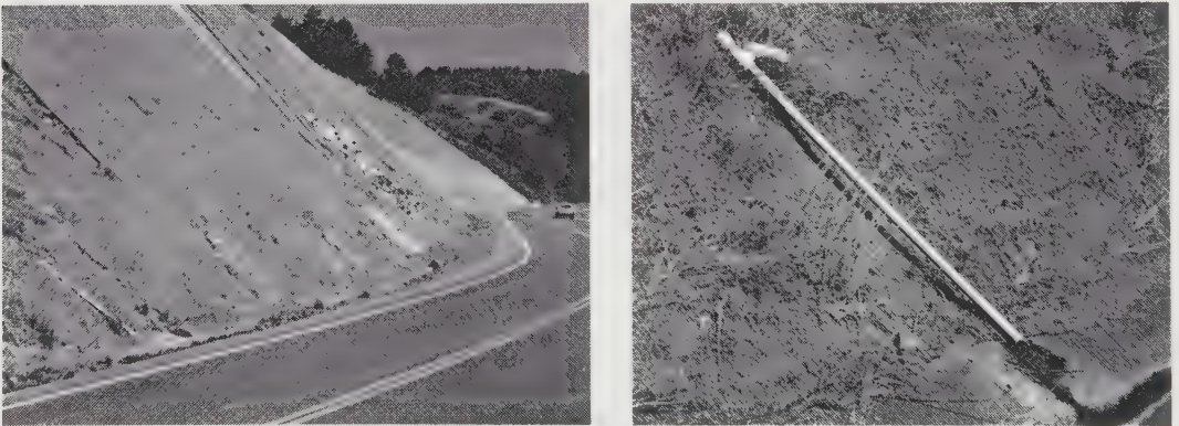
Figure 14.41 A series of horizontal drains in a cut slope along a highway. The close-up view shows one of the drains exiting the slope and discharging into a swale. This drain has a slow but continuous flow, as evidenced by an accumulation of algae at its discharge point.
