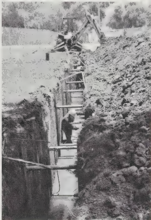
Figure 3.15 This exploratory trench was dug by the backhoe in the background, and has been stabilized using aluminum-hydraulic shoring. An engineering geologist is logging the soil conditions in one wall of the trench. In this case, the purpose of the trench is to locate a fault.
