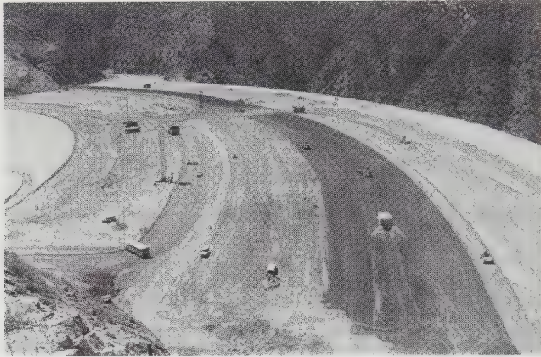
Figure 15.5 Seven Oaks Dam under construction. The dark zone in the center of the dam is the zone 1 core material. It is surrounded by the other zones, per the cross-section in Figure 15.4. The downstream face of the dam is visible on the left side of the photograph.
