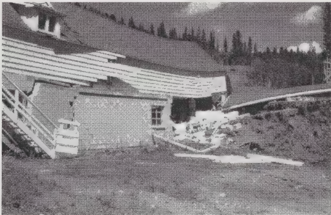
Figure 20.16 Culligan's Blarneystone Ranch, Montana. Surface rupture during the 1959 Hebgen Lake Earthquake passed through this building, causing part of it to completely collapse (seen behind the scarp) and severe damage to the remaining section (on the left). This earthquake produced displacements up to 5.5 m (18 ft), which is far more than any building can accommodate. (Earthquake Engineering Research Center Library, University of California, Berkeley, Steinbrugge Collection)
