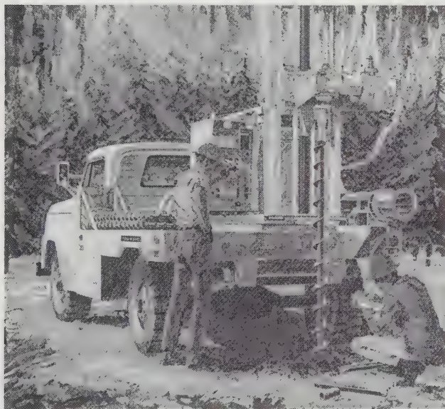
Figure 3.6 A crew drilling an exploratory boring using a truck-mounted flight auger. These augers typically have an outside diameter of 120–200 mm (3–8 in). (Foremost Mobile Drilling Co.)
