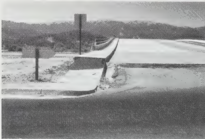
Figure 11.2 The approach fills adjacent to this bridge in California have settled. However, the bridge, being supported on pile foundations, has not. Note the abrupt change in grade in the sidewalk, and the asphalt patch between the two signs. This photograph was taken about twelve years after the bridge was built.
