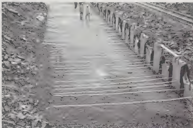
Figure 16.26 Reinforced earth walls consist of precast concrete facing panels and steel or polymer reinforcing strips that extend into the retained soil. This wall is under construction (The Reinforced Earth Company).
