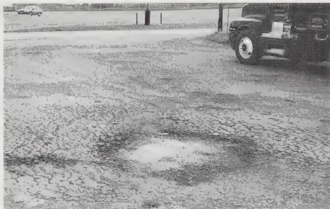
Figure 18.4 The soils beneath this asphaltic concrete pavement in New York became wet and soft during the spring thaws. As a result, these soils failed under the weight of the heavy trucks that use this site. The pavement is now in very poor condition, with extensive alligator cracks and potholes.
