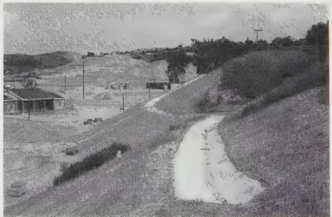
Figure 14.38 Typical surface drainage facilities on a cut slope. This concrete terrace drain captures surface water and carries it to a safe discharge point.
