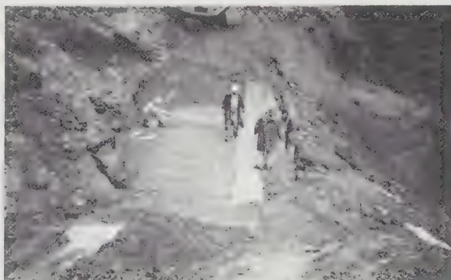
Figure 16.28 An MSE wall under construction using galvanized wire mesh as the tensile reinforcement and rock-filled cages called gabions for the facing (Federal Highway Administration).
