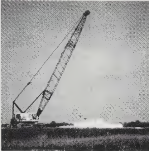
Figure 19.6 This crane is densifying the soil using dynamic compaction. It has just dropped a large weight onto the ground (GKN Hayward Baker, Inc.).
