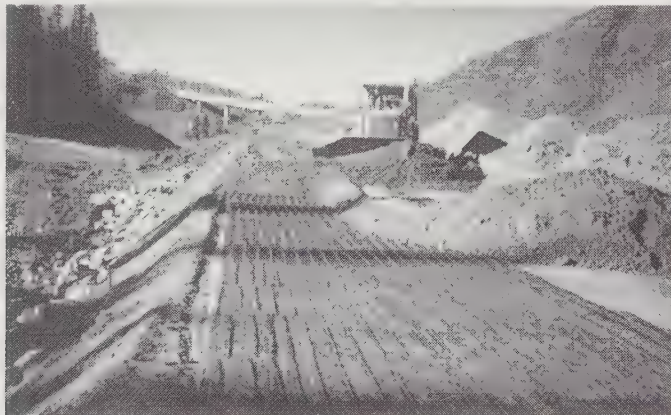
Figure 19.10 Geogrids being used to reinforce a fill for a highway. Multiple geogrids are used, each separated by a layer of soil. (Courtesy of Tensar Earth Technologies, Inc., Atlanta, Georgia, USA)
