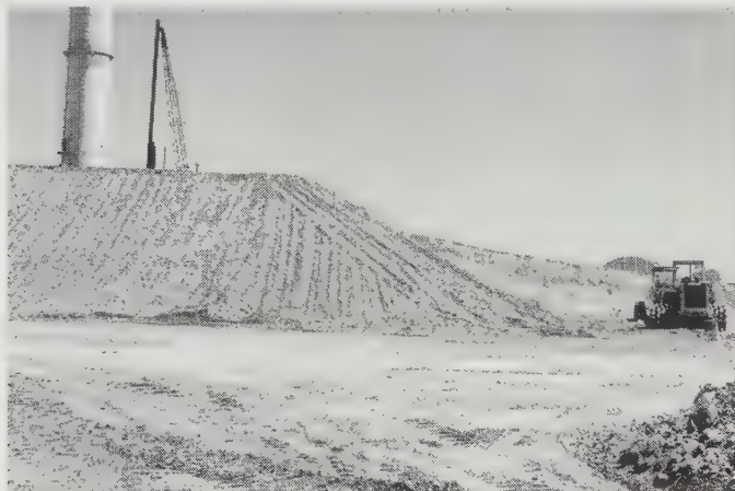
Figure 19.1 This surcharge fill will remain in place until the underlying soils have settled. The smokestack and crane in the background are located behind the fill.
