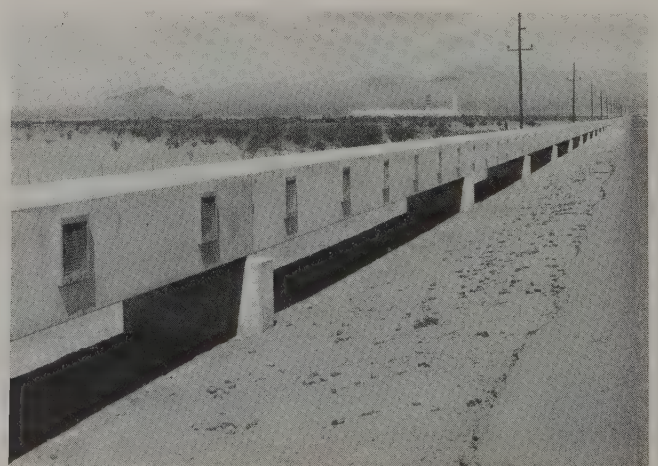
Figure 5.44. Belt conveyor in concrete support housing.
