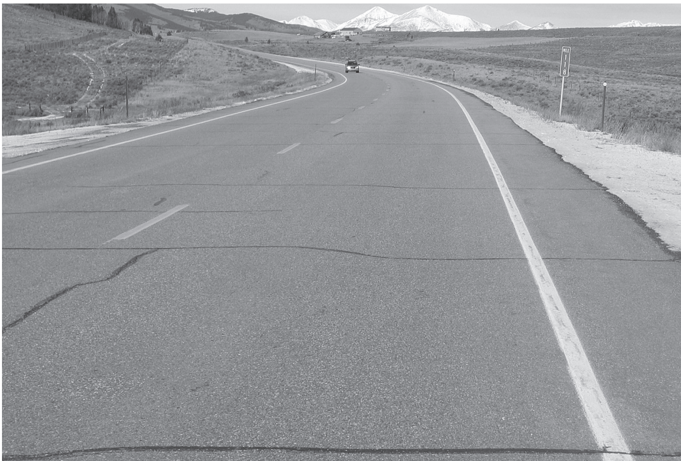
FIGURE 10.18 Transverse (Thermal) Cracking
