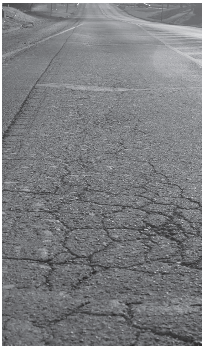
FIGURE 10.13 Load-Associated Cracking (Alligator Cracking)
